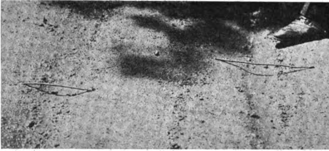
Narrow Ruts, Three Inches Deep, in Macadam.
